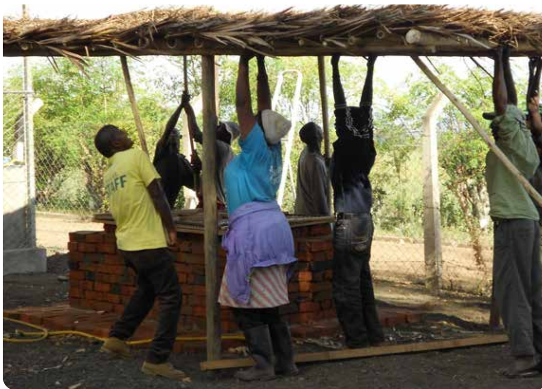
Raising the roof at the Zero Energy Cool Chamber training in Tanzania - Photo: Lisa Kitinoja/Postharvest Education Foundation
