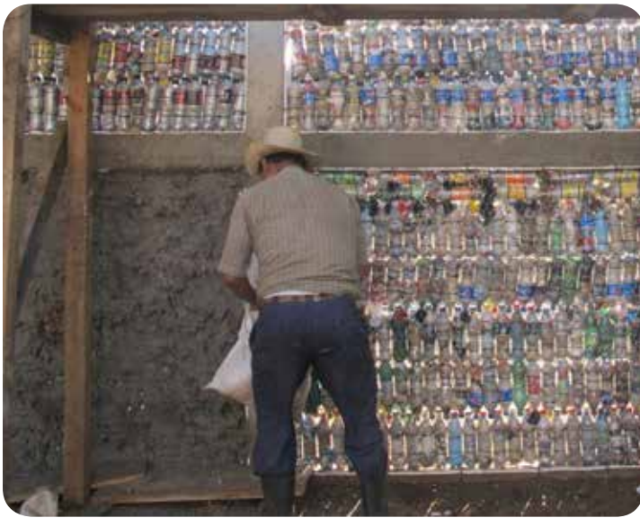
Building a bottle brick (“ecoladrillo”) structure in Chipila, Guatemala; bottles filled with inert waste are affixed to a mesh backing and covered with a cement veneer - Photo: HugItForward.org
