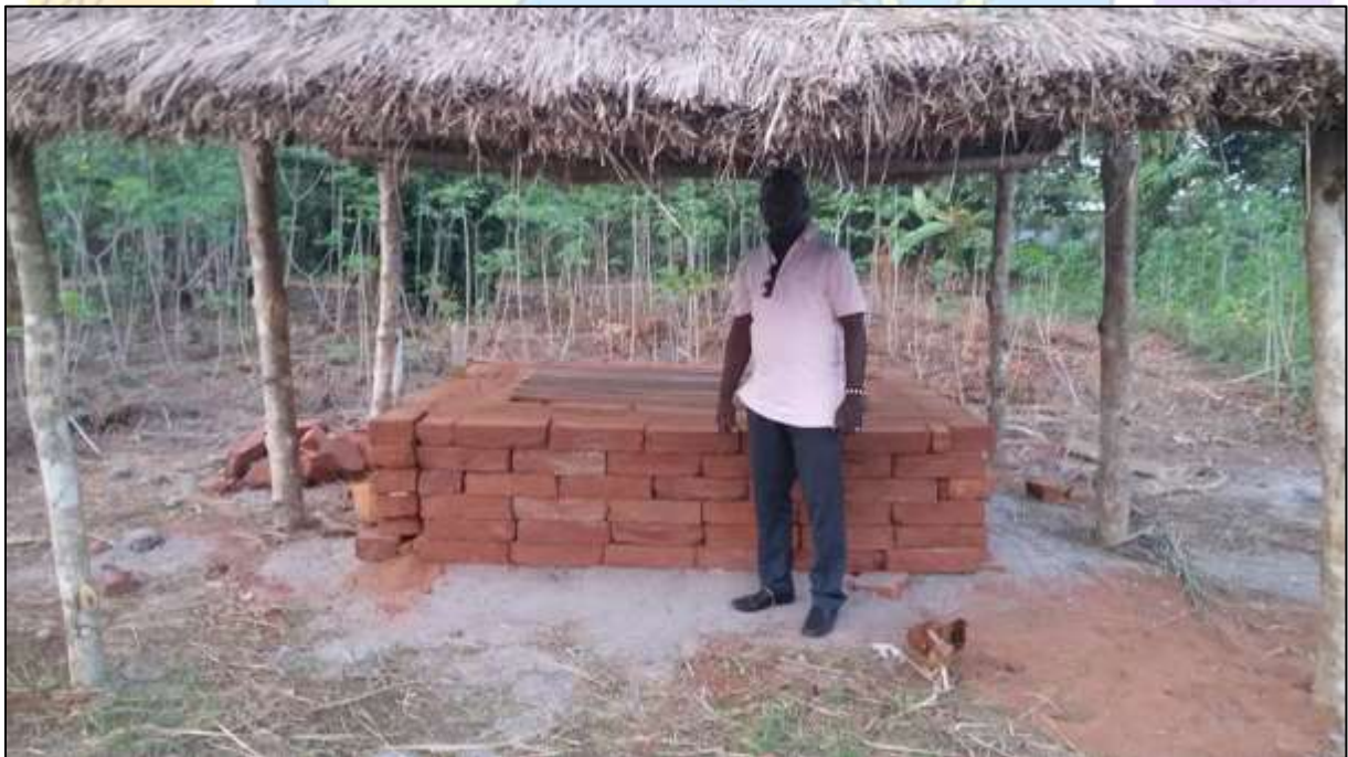
Photo of a Zero Energy Cool Chamber (ZECC) being constructed on a farm in Benin by Guy Kodjogbe, PEF board member
