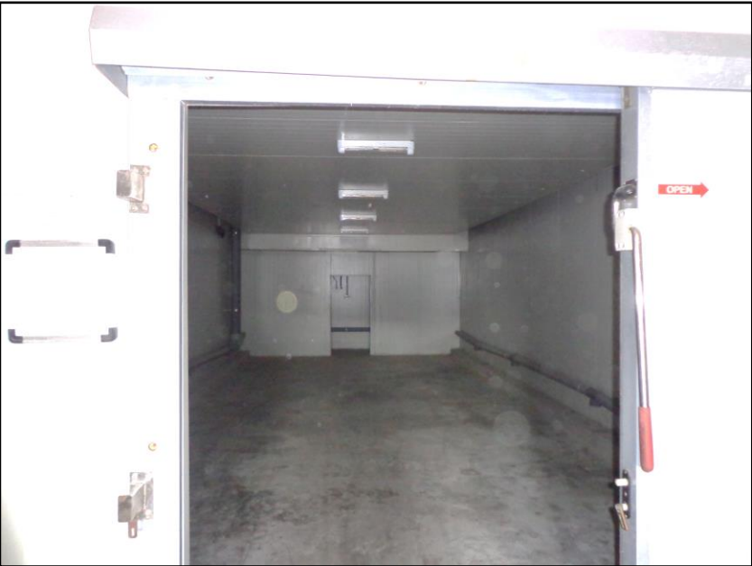
Cold storage/Ripening room
