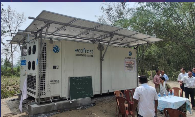
Solar powered cold rooms in Assam, India
